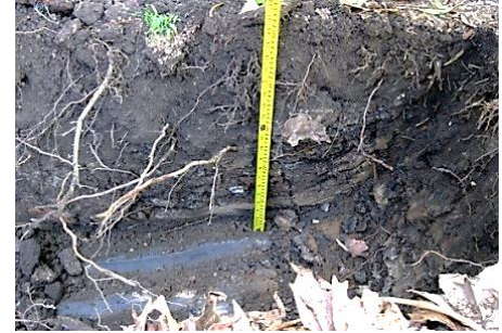
b) Example of a cut
